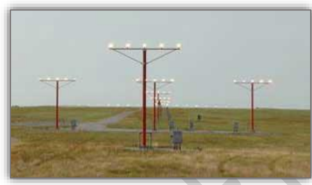
FAA, Lighting System – Medium Approach Light System with Runway Alignment Indicator Lights (MALSR), 2019.
